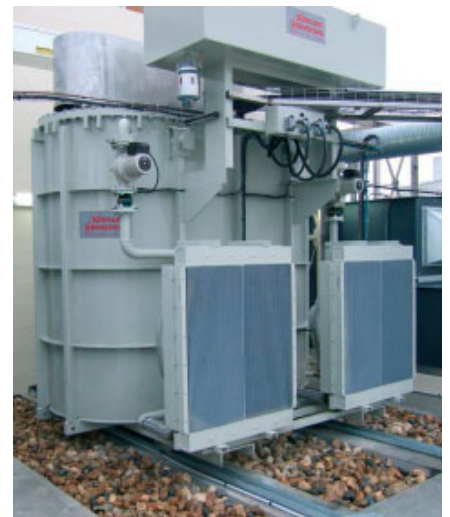
Stationary Oil Cooling for a power transforming plant, Bernard & Bonnefond
