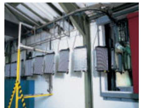
Electrostatic paint line
